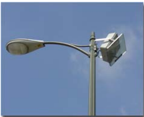
Closed-circuit camera mounted on a light post.
